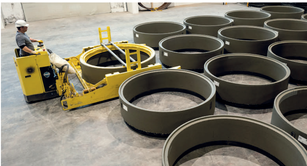
Fresh products are carefully transported to the curing area using an electrical cart for transportation and a set ring manipulator.
