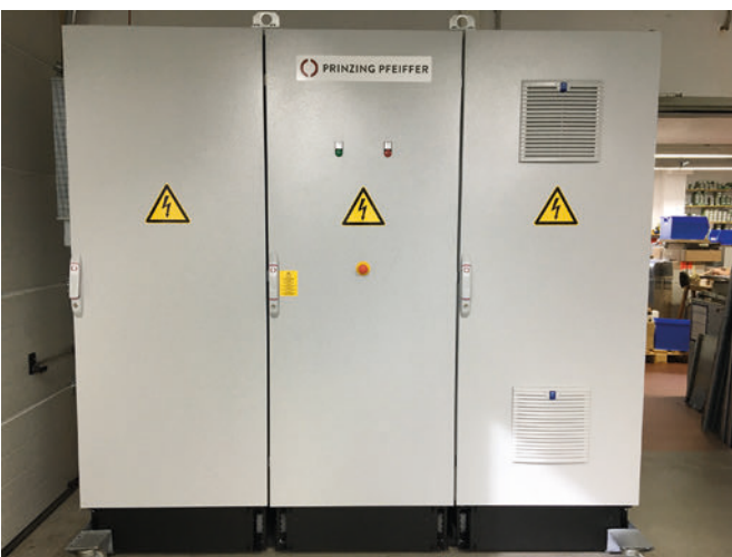
Electrical control system for the Radial Press RP 1230, built in a 3-door control cabinet including the latest worldwide proven Siemens Simatic S7 PLC technology
