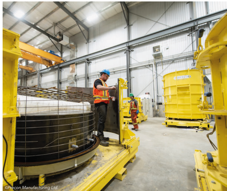
Setting up the channel, climbing aids, and reinforcement in the wall and floor.
