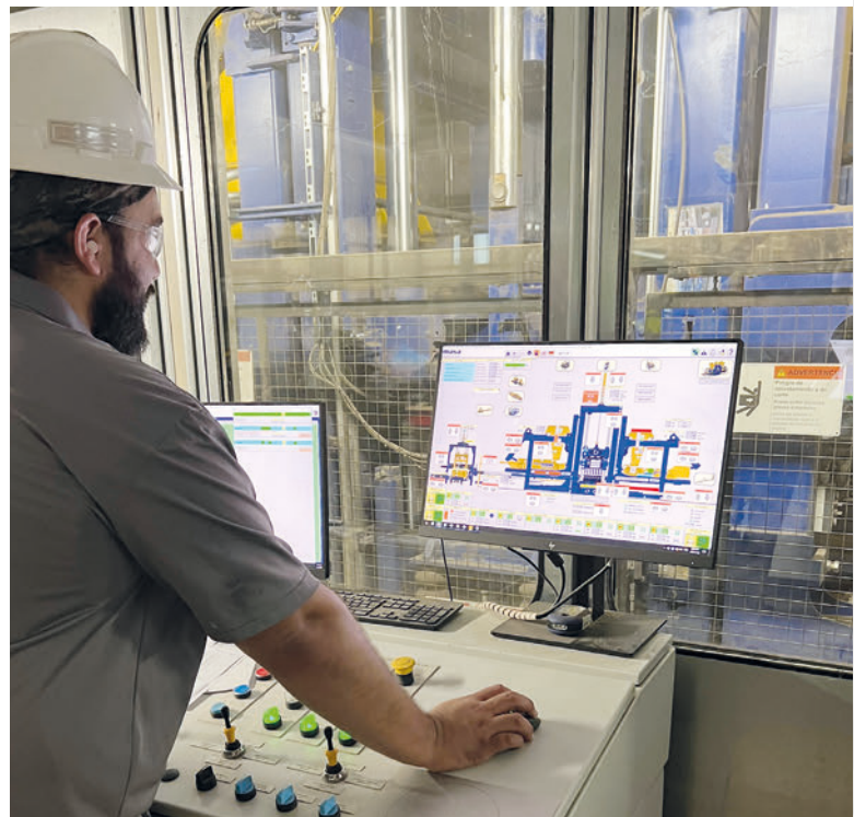
Real time animated controls allow the operator to see all processes at any stage from multiple screens.
