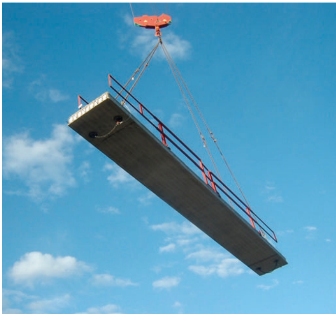
The indoors produced hollow core elements are then transported to the construction sites and installed in a short period of time.
