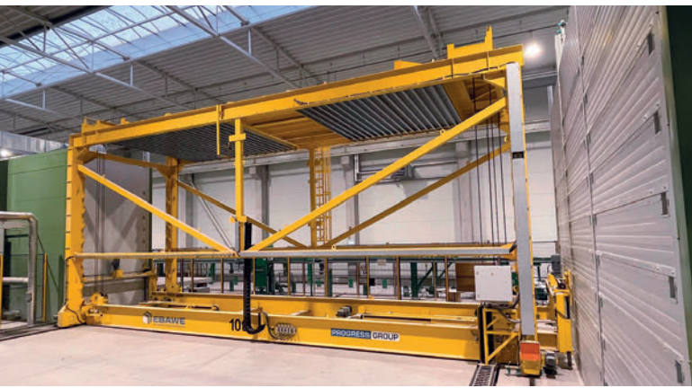
The pallet stacker is stacking the casted elements to the curing rack.
