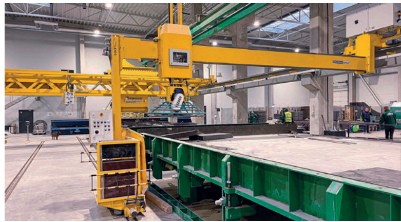
After the curing of the concrete surface the next phase is fine smoothing with a power trowel.
