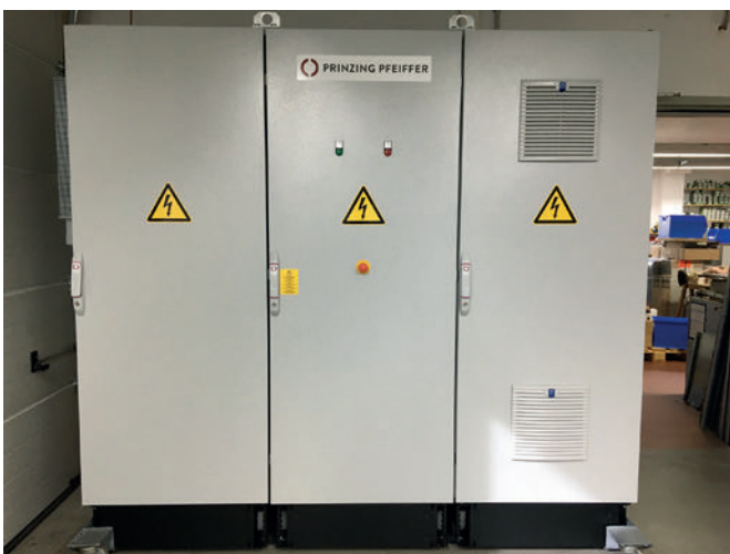
Electrical control system for the Radial Press RP 1230, built in a 3-door control cabinet including the latest worldwide proven Siemens Simatic S7 PLC technology
