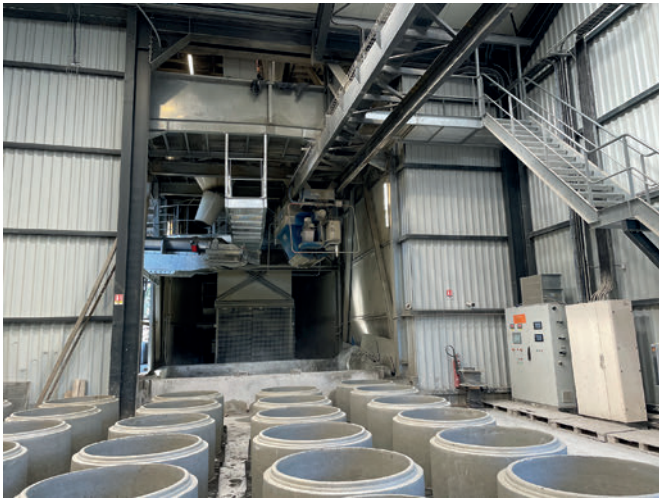
The Teka mixing plant produces the concrete for all the production areas
