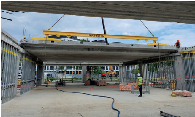
The prefabricated elements can be implemented faster and safer at the building sight.
