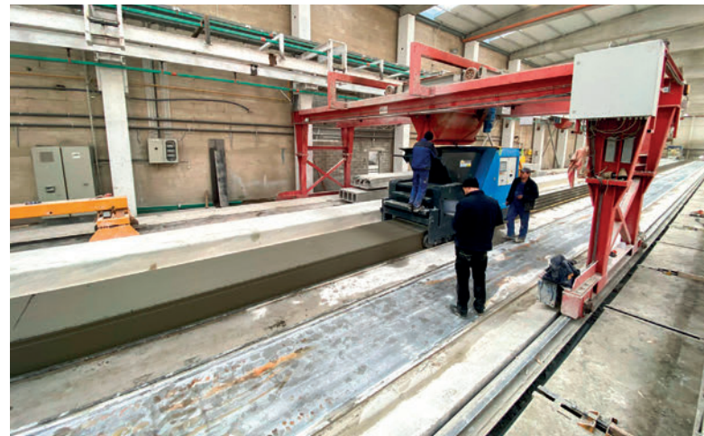
With a professional installation, the extruder was up and running within one day.
