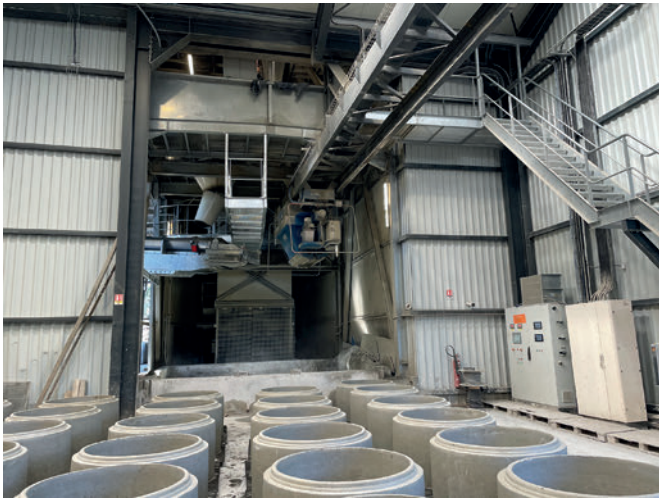
The Teka mixing plant produces the concrete for all the production areas
