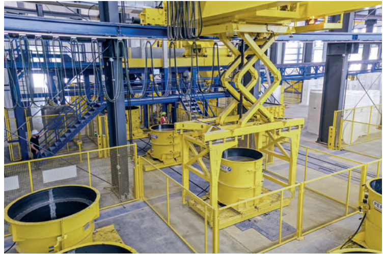
Continuous processing of SCC constitutes a vital basis for efficient operation of an industrial wet cast production plant.
