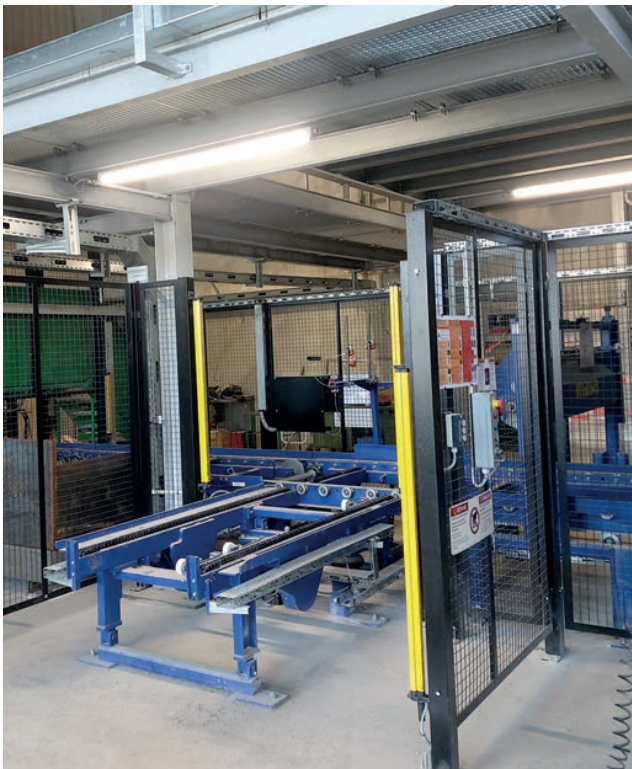
Control station for reliable quality control
