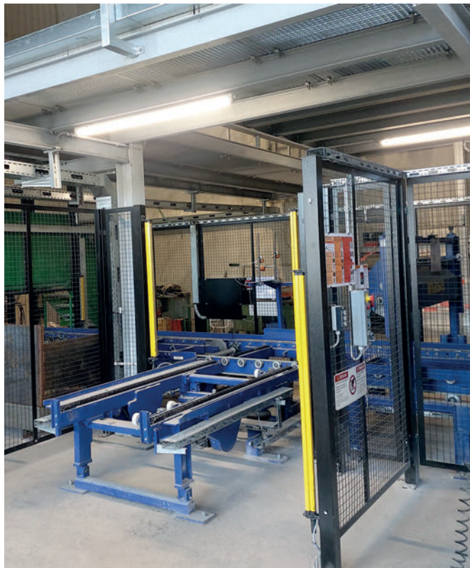
Control station for reliable quality control
