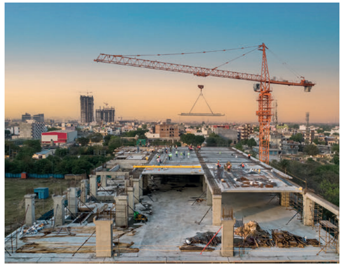
Building with precast elements reduces material needed, manpower and mistakes on site - all while increasing quality.
