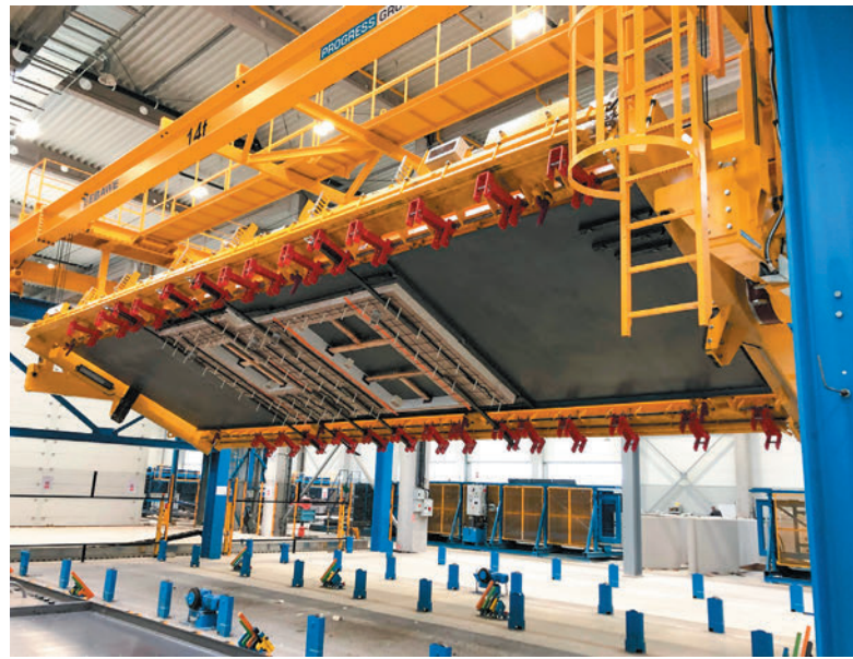
The turning equipment from Ebawe Anlagentechnik is fully automated and working precisely to the millimetre.
