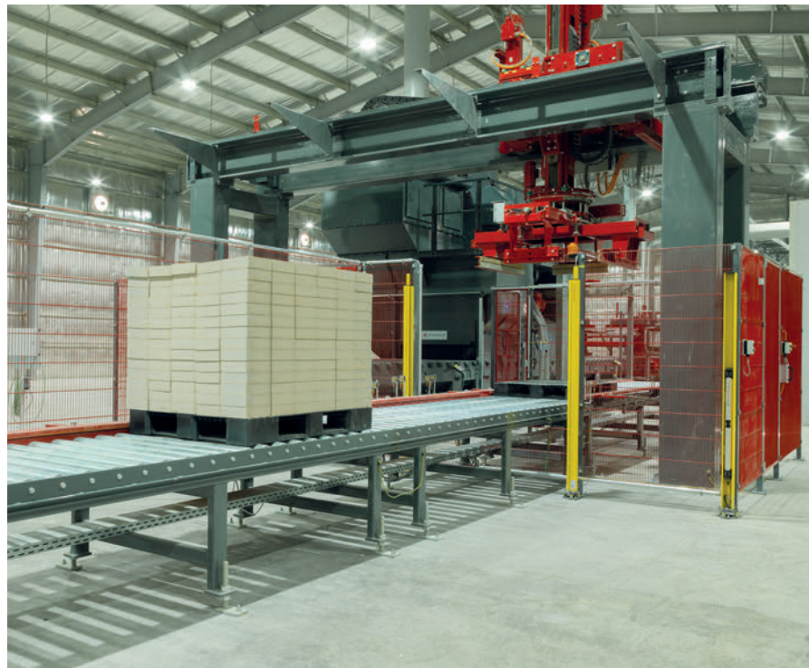
The stone packages being finished are transported by the heavy-duty conveyor to the LPU layer stacker.
