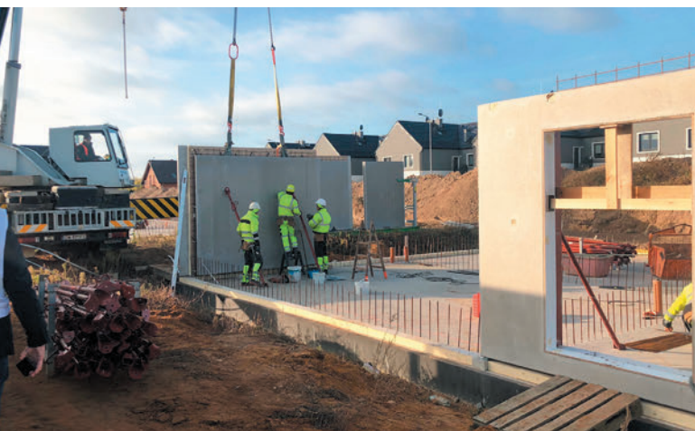
The fast assembly on site is done by a well-trained and professional team, which knows how to work with the different prefabricated precast elements.
