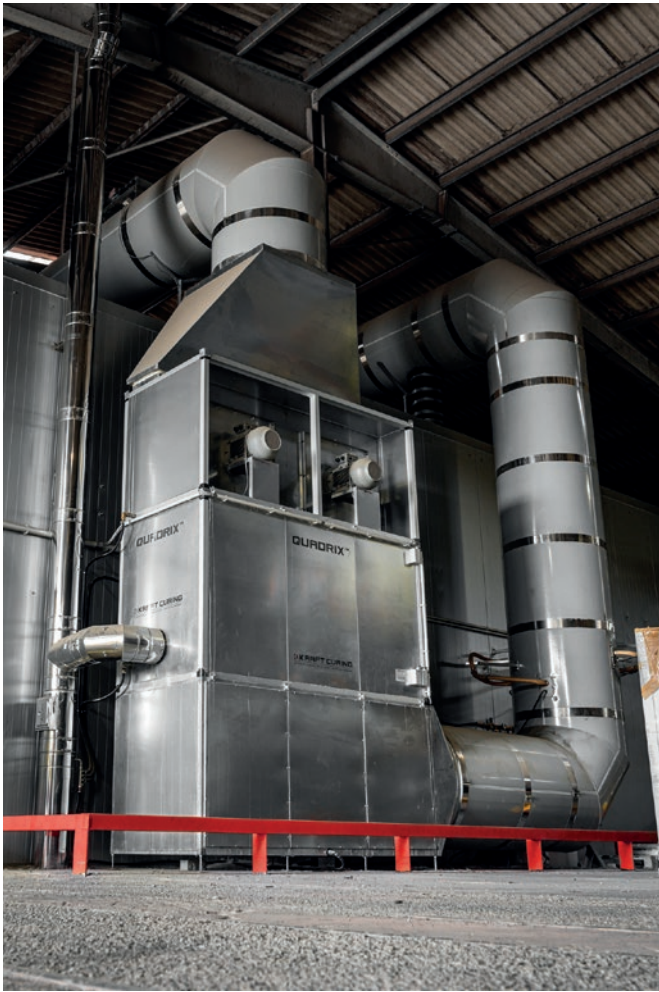
Systems technology possible with a wide range of energy sources
