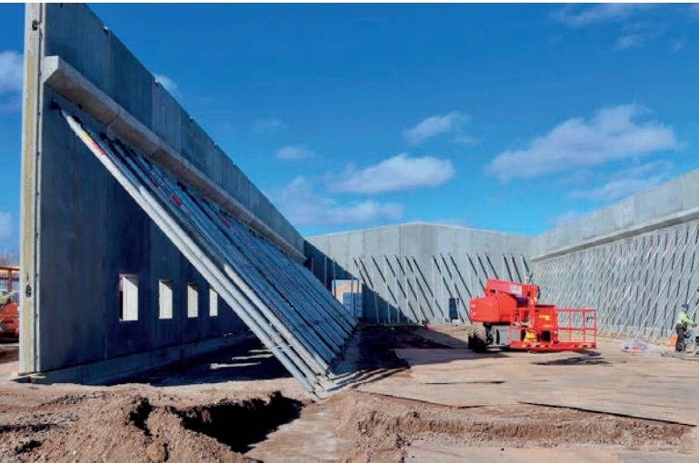
The construction of the hall and the installation of the machine could be finalised in the summer of 2021.
