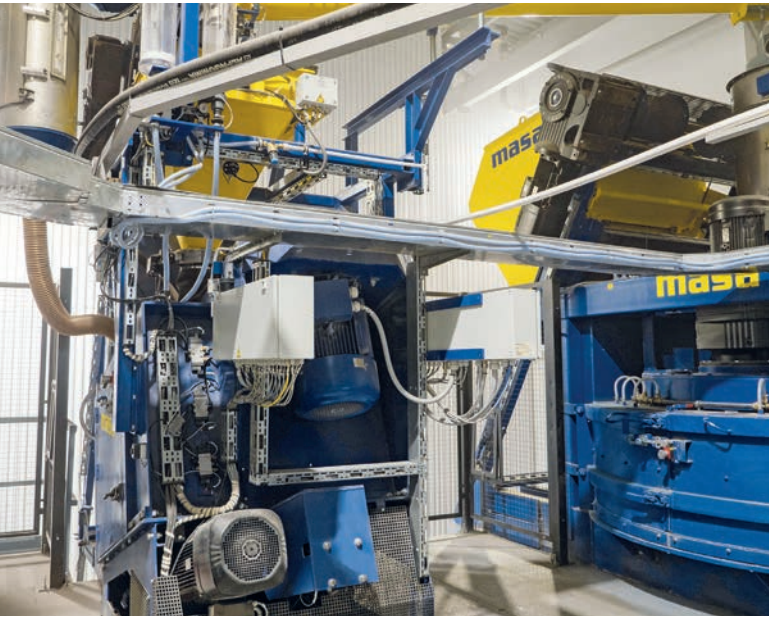
The mixing area includes a Masa mixer S 350/500 (left) for face mix concrete and a Masa mixer PH 1500/2250 for main mix concrete
