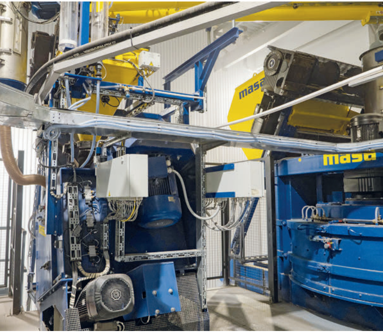
The mixing area includes a Masa mixer S 350/500 (left) for face mix concrete and a Masa mixer PH 1500/2250 for main mix concrete
