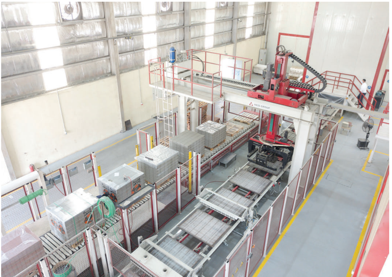
The packets of blocks are formed on the 28-m long slat conveyor arranged in parallel and then transported outdoors in cycles.
