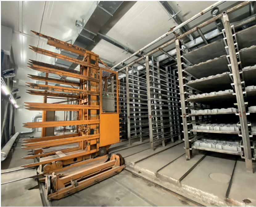
View inside the curing chamber with the Quadrix pipe systems on the ceiling and floor.
