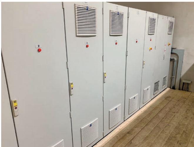
Everything on its place in the new, air-conditioned, and dust-protected switch cabinet rooms
