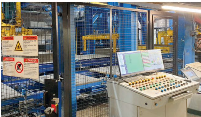
The new control panel for the area of return transport and remodeling.
