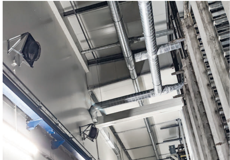
Internal ducts maintain the right climate inside the chamber
