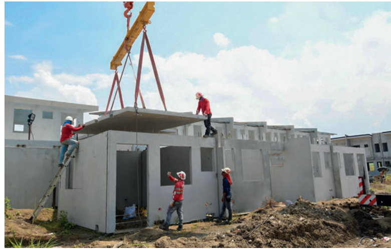
The precast elements used are 100 mm wide solid walls all around both floors as per minimum code requirement. The 120 mm solid slabs are provided as one piece.
