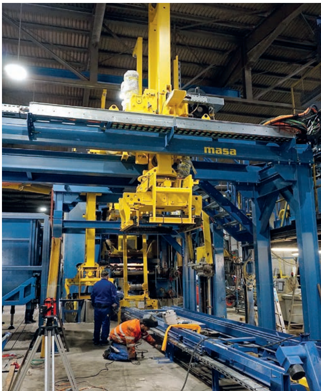
During the reconstruction phase: Assembly of return transport, Shifter III and IV as well as Cuboter
