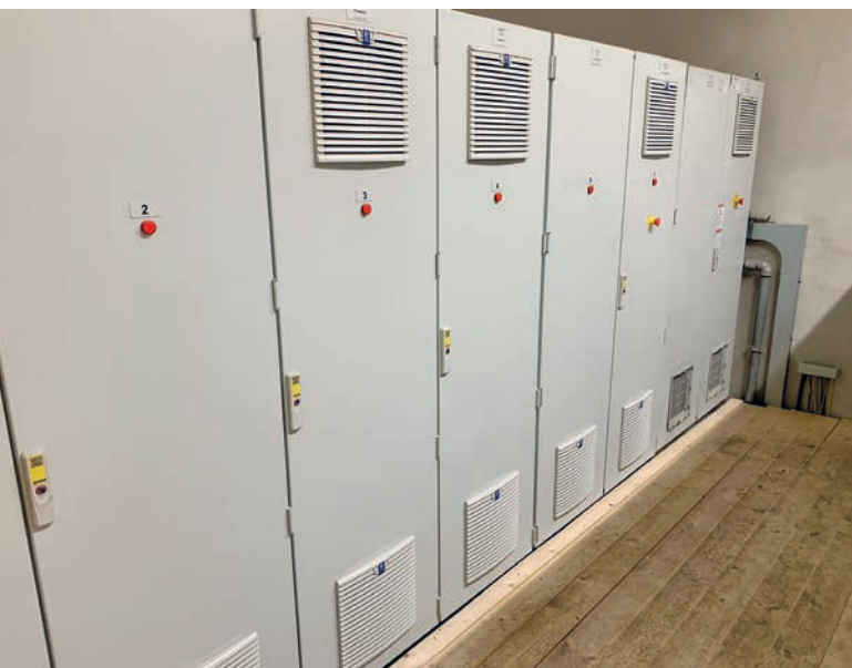
Everything on its place in the new, air-conditioned, and dust-protected switch cabinet rooms
