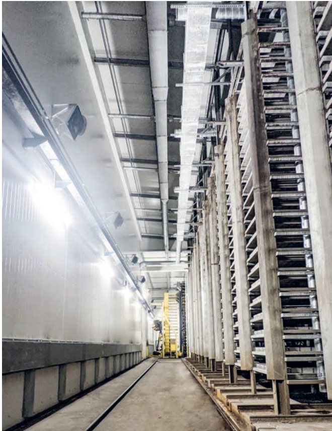
The transfer table aisle was also insulated; lights and fans were installed
