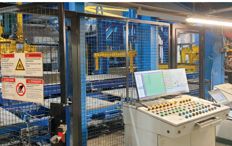
The new control panel for the area of return transport and remodeling.
