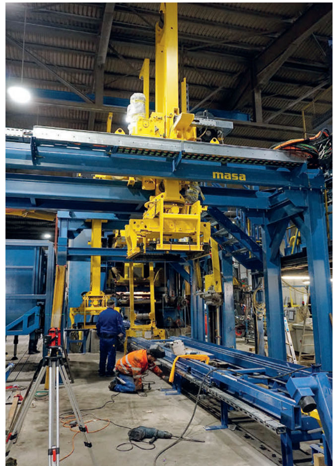
During the reconstruction phase: Assembly of return transport, Shifter III and IV as well as Cuboter
