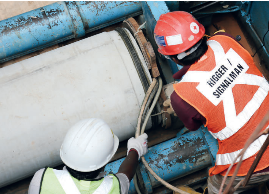
Installation of Perfect Pipe jacking pipes in the first project of its kind implemented in Singapore—this was reported on in CPI 2/2016.
