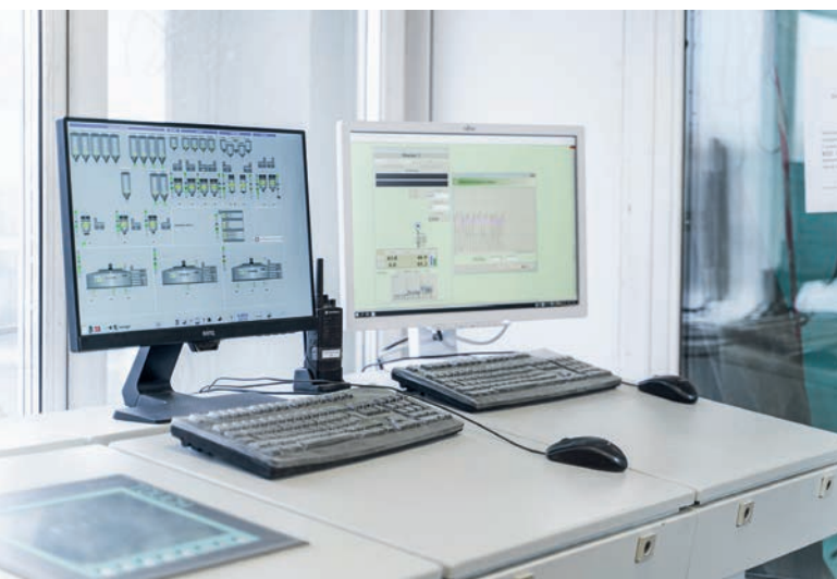
The control centre of the concrete mixing and transport plant
