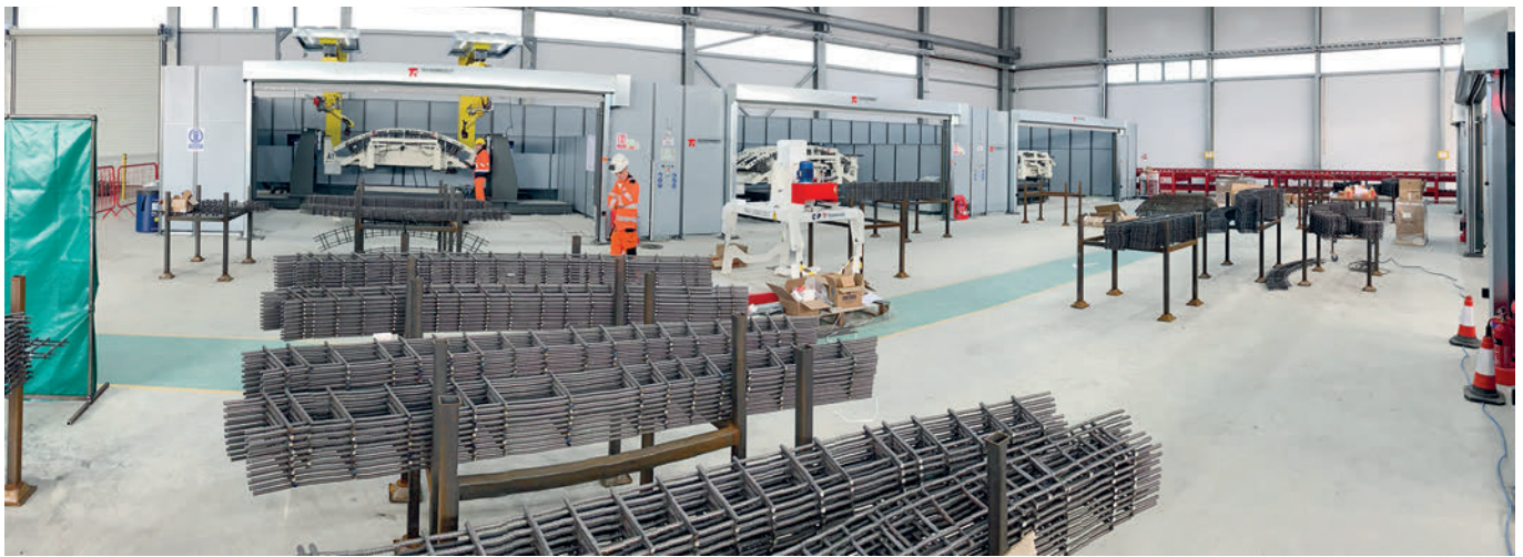
The prefabricated ladders are welded together with the reinforcement meshes by the welding robots (visible in the background) to form the finished cage for tunnel elements.
