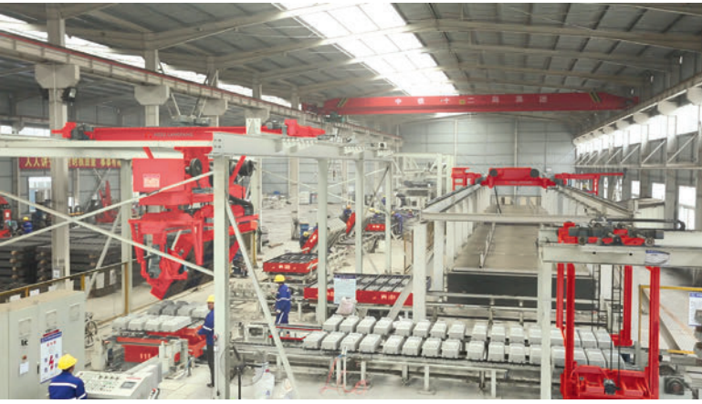
Figure 2: Modern carousel line system - First project of China Railway 12 th Bureau, Lanxin Daban City
