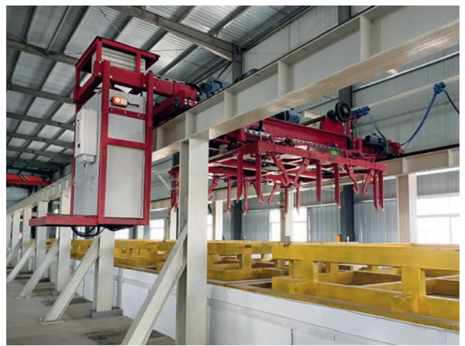
Figure 4: Mold stacking device for handling of molds and curing pit covers
