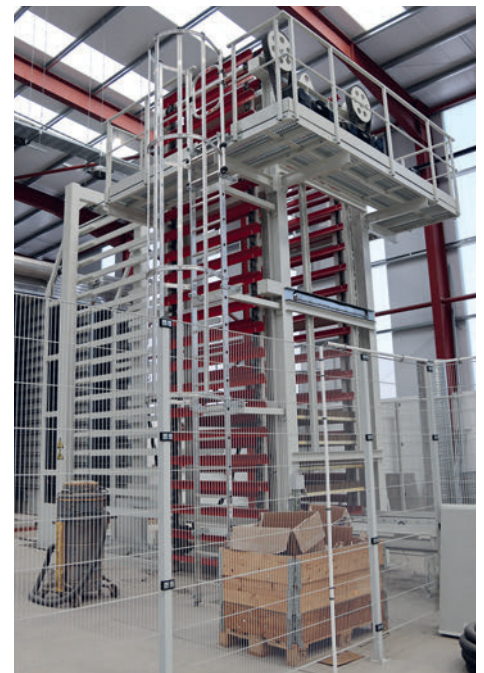
There is one buffer car behind the elevator and one in front of the lowerator on the wet side and on the dry side respectively, each with 17 tiers (double discharge system) and 14 tons of capacity.
