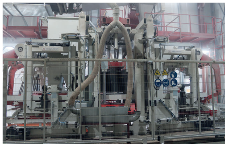
The Hess RH 1500-4 MVA concrete block machine is the heart of the production plant.
