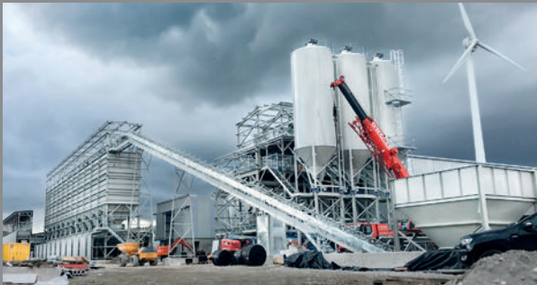
Rapid International's batching and mixing plant in the assembly phase: on the right the mixing tower with the three 150-ton cement silos, on the left the units with a total of 29 storage bins for aggregates and sand.
