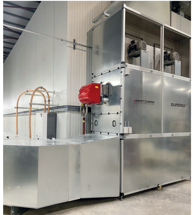
The ideal climate in the individual chambers is ensured by the latest-generation Quadrix Ultra concrete curing system from manufacturer Kraft Curing Systems.
