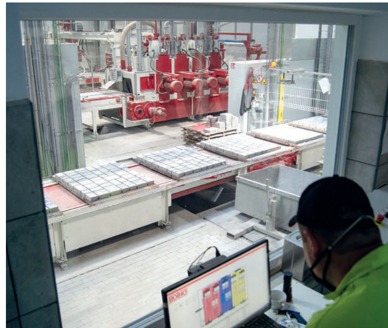
View from the control cabin towards the dry side; in the background is the SR Schindler curling machine
