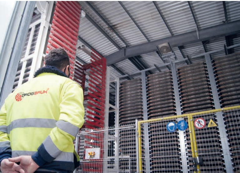
Lowerator and finger car unit are located within the Rotho large chamber rack system with a Pro Cure heating system
