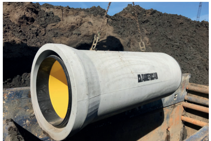
American Perfect Pipe is installed in Nebraska. A corrosion-protected flexible pipe system is produced immediately after the pipe has been installed.
