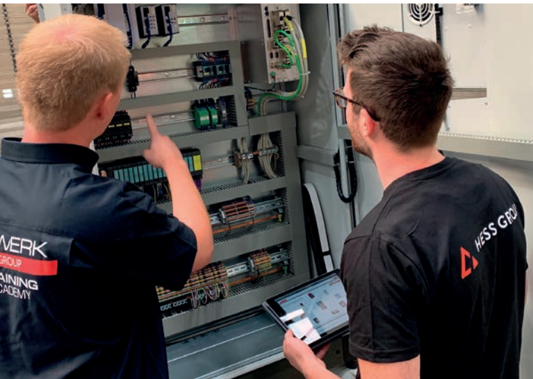
Introduction to the functionality of the control cabinet
