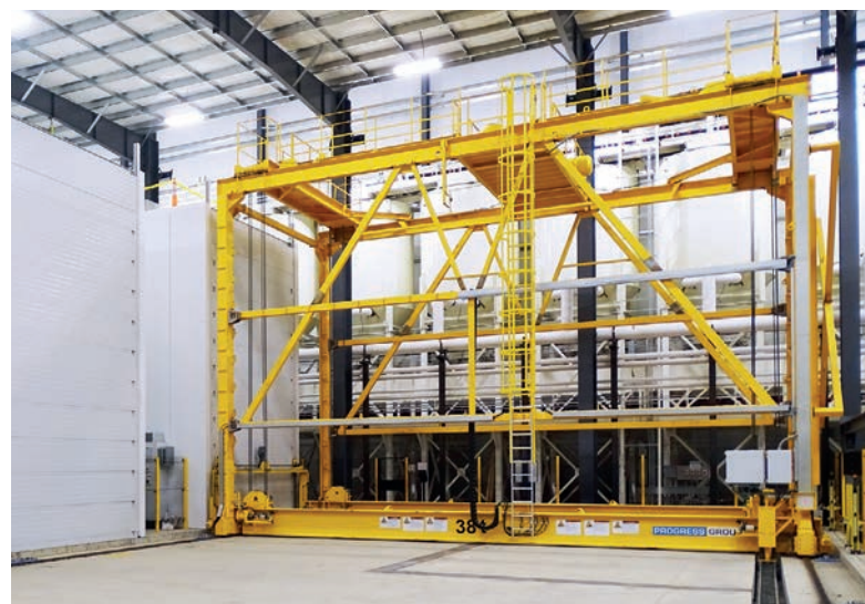
The pallet stacker serves the two racks and stores and retrieves the pallets with the freshly concreted solid wall elements.
