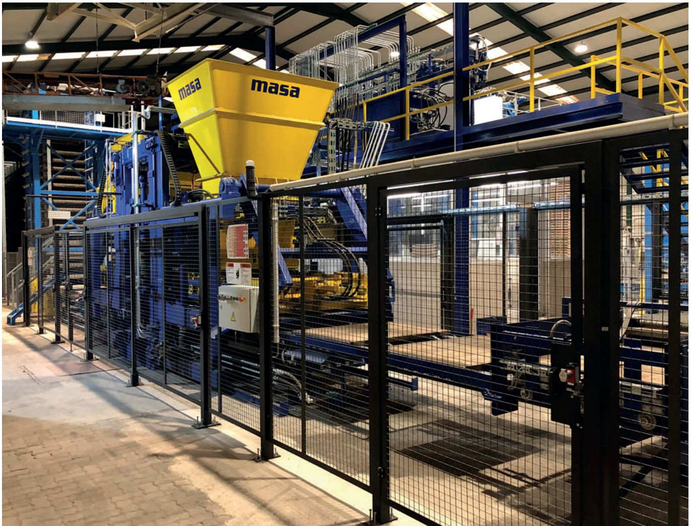
The new Masa L 9.1 is the heart of the plant.
