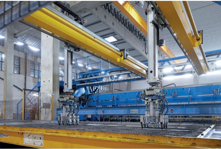
The reinforcement was also automated to the greatest possible extent in the new factory for double walls and precast slabs with in-situ topping in Könnern. The Wire Center laying robot places longitudinal and transverse bars as well as the lattice girders into the shuttered pallets with two robot arms.
