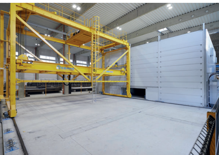
The stacking rack offers space for 36 pallets and is served by a lifting transfer table.
