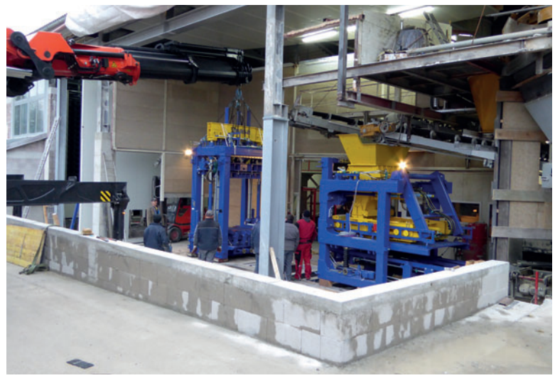
The compaction unit of the new Masa XL 9.1 is installed.
