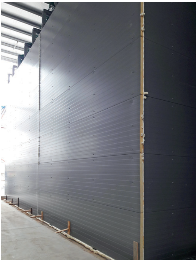
Obsessed with detail: Kraft fitters foam all joints between the sandwich panels for an airtight enclosure prior to affixing the flashing to prevent any heat loss. This detail eliminates the formation of condensation and prevents corrosion while reducing energy costs.
