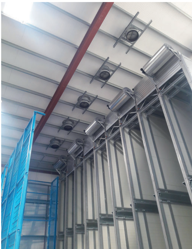
Nine independently controllable individual chambers form the new curing system for concrete slabs from the radial press and allow Kilsaran maximum flexibility in production.
