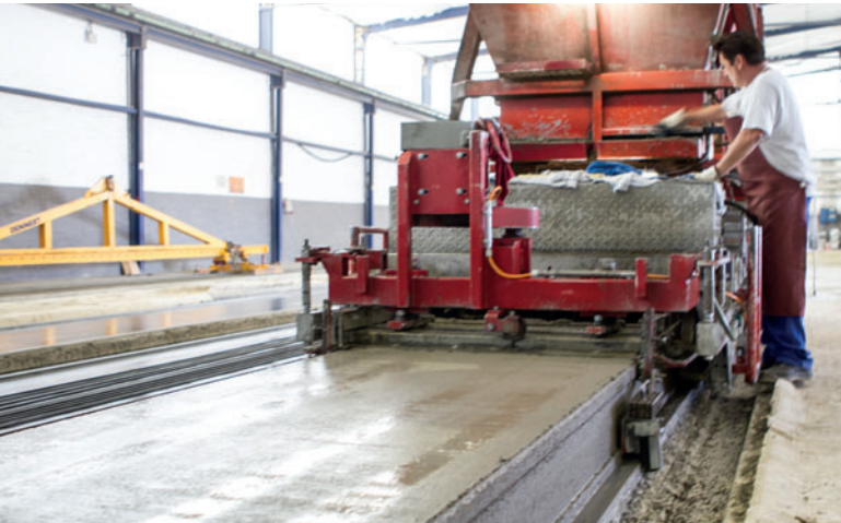
In addition to the saw for cured prestressed hollow-core slabs, Dennert uses the S-Liner slipformer from Echo Precast Engineering on its five production lines (Photo: Dennert).
