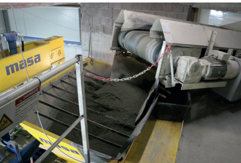
Belt feeding of the main mix concrete silo.
