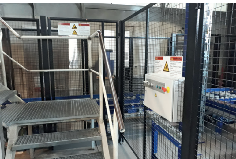
Security is a major priority at St. Georgen.
