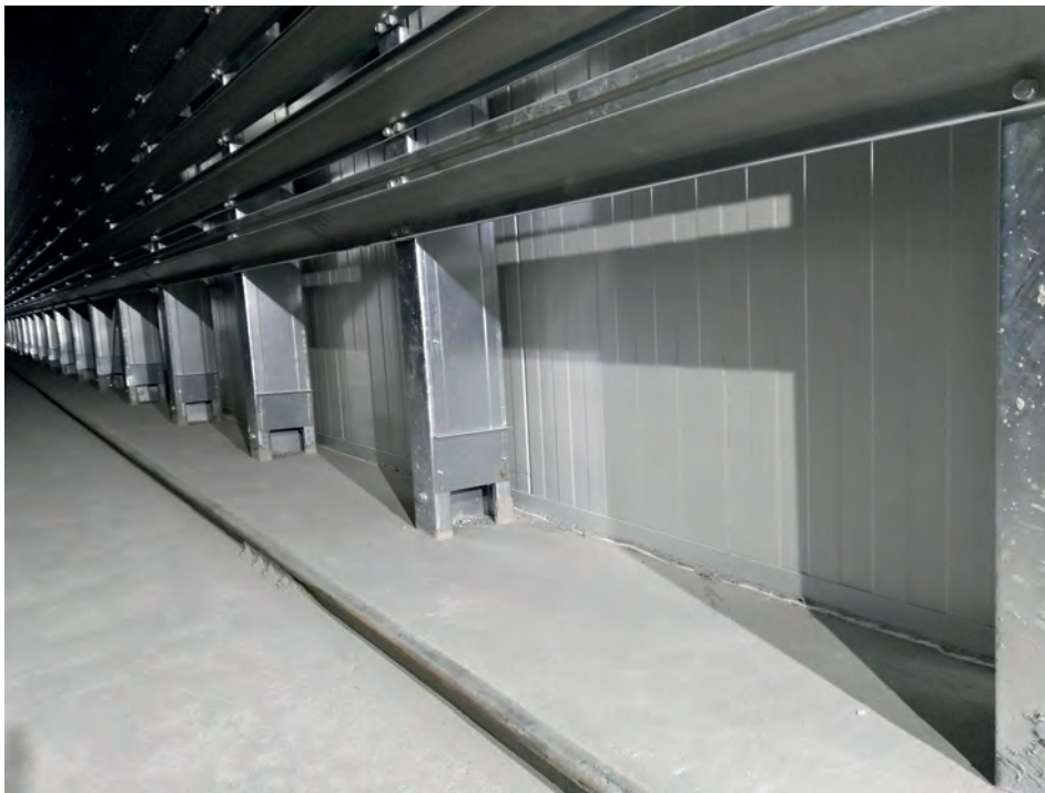
Fig. 5: Every single perimeter column of the Kraft rack functions as an air duct, heating the chamber floor, thus avoiding condensation and eliminating corrosion. (Picture: Kraft Curing Systems)
