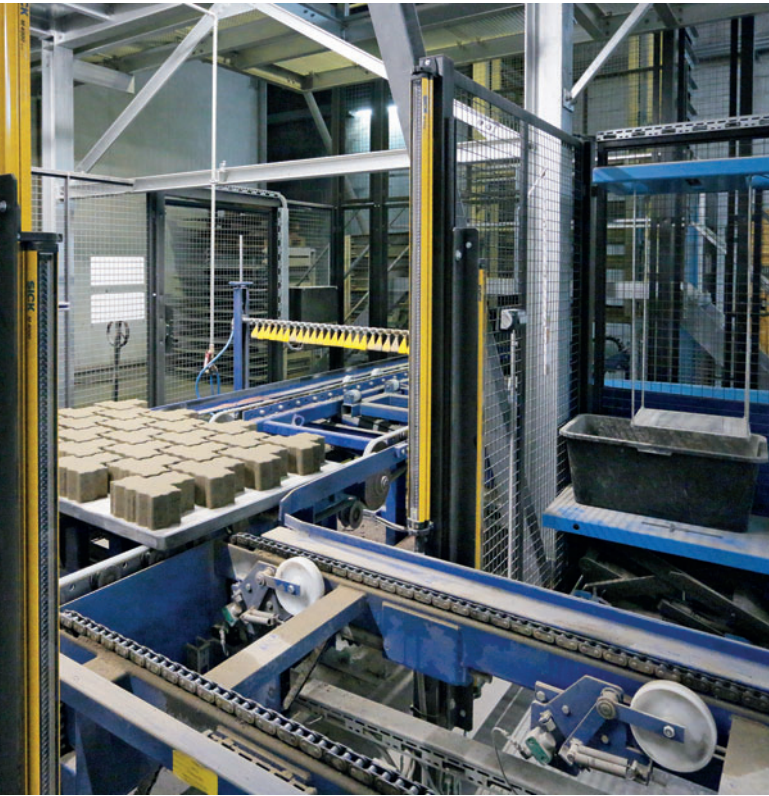
Modular V-belt conveyor system with quality control station
