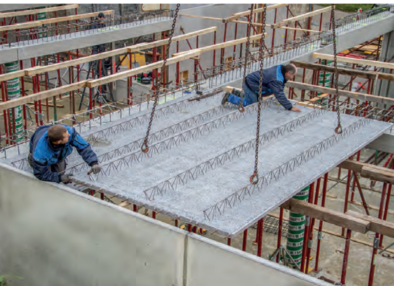
In the modern pallet circulation plant from Ebawe Anlagentechnik, Jungwirth manufactures precast slabs with in-situ topping and double walls with and without insulation.
